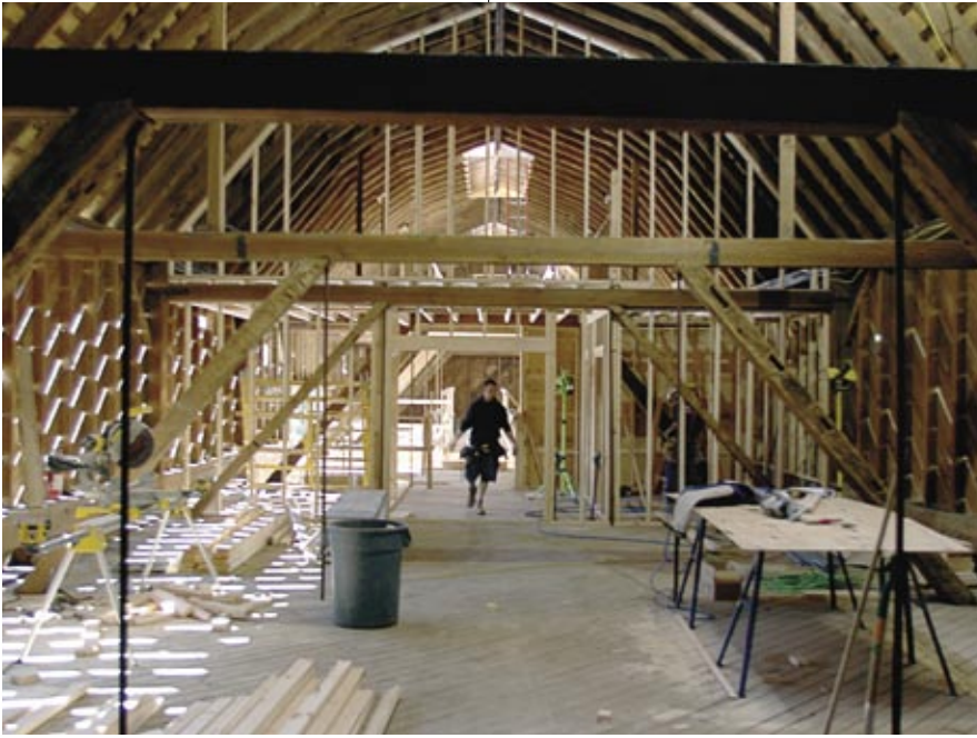
The renovations to the second floor of the Johnson Education Center. Formerly the hayloft, this area will become the RWJ Auditorium. The original architecture, including the exposed timber and wood framing and sheathing, will be retained.
